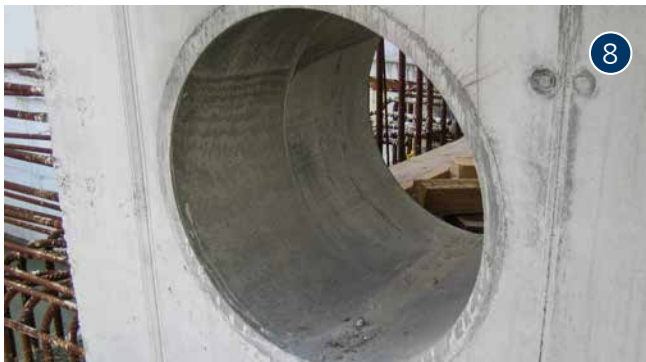
FZR400/300 installed in a water treatment plant
