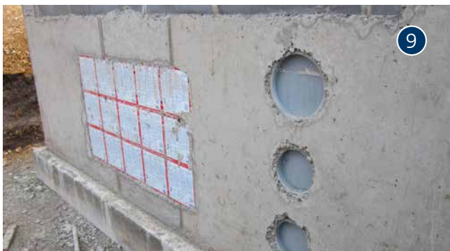
ZVR150 and ZFR200 concreted in the wall next to HSI150 3x5 package
